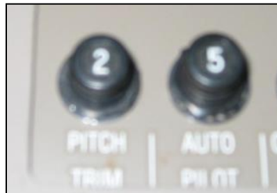
Autopilot and Electric Trim Circuit Breakers
